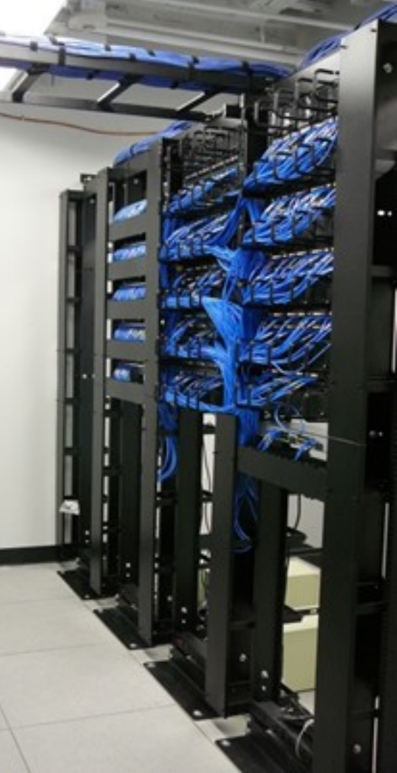
Image: Telecommunications Closet
